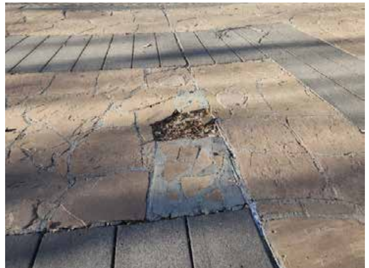
Figure 14. Deteriorating surface materials.
