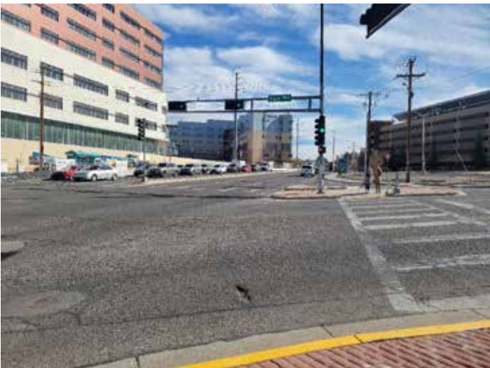
Figure 7. Crosswalks at Lomas & Yale in poor condition.
