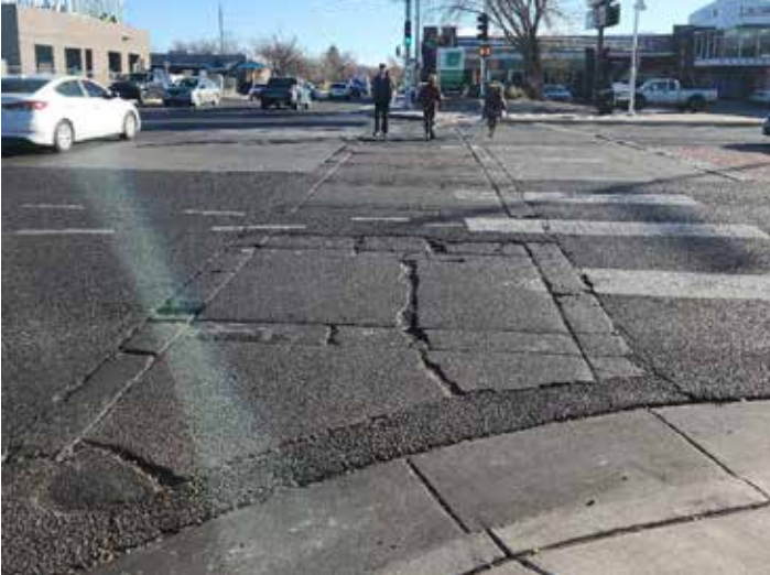
Figure 5. Crosswalk at Central & Girard in poor condition.
