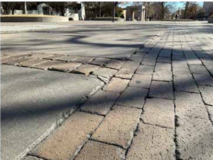
Figure 13. Brick pavers and raised concrete edges are hazards.
