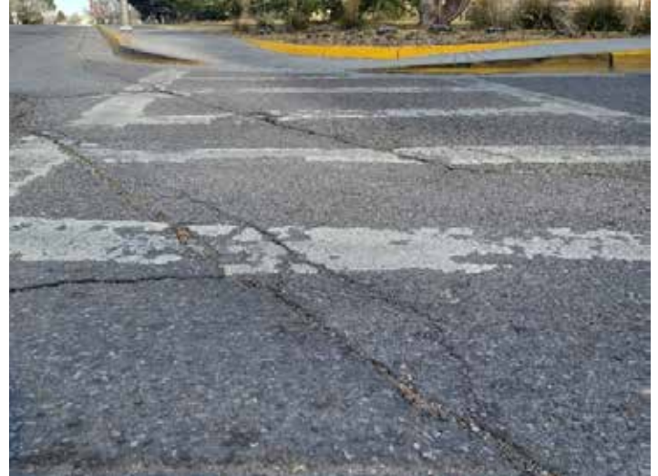
Figure 6. Uneven surfaces conducive to trip hazards.
