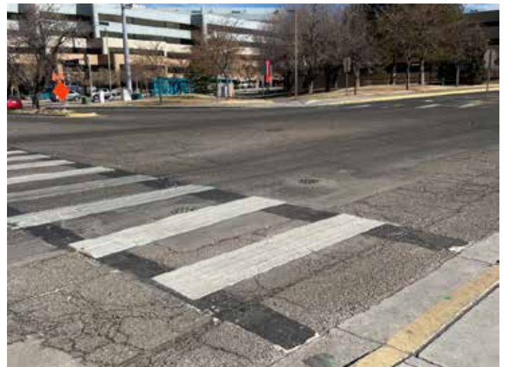
Figure 8. Poor crosswalks at Stanford & Campus.
