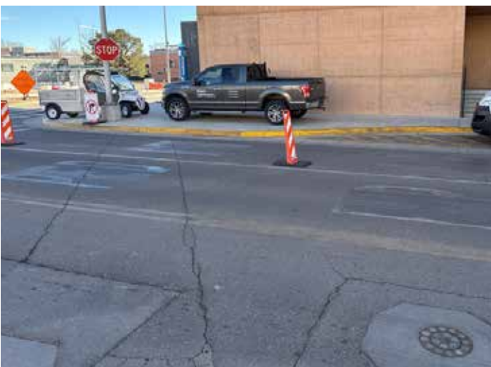
Figure 15. Surface markings promoting MMV safety is fading.
